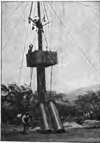
Fig. 312—Showing Workmen's Cage Which is Carried to the Top During the Process of Erection.
